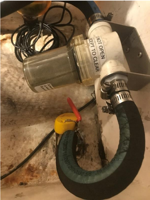
Seawater Thru Hull to Cool Engine
