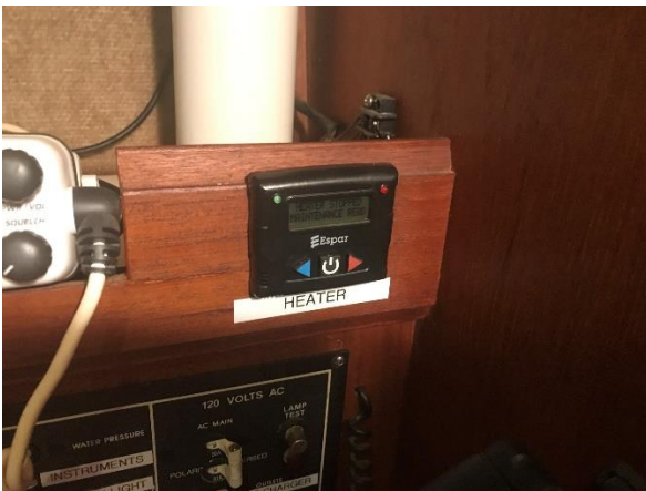
Heater Control above Electrical Panel
