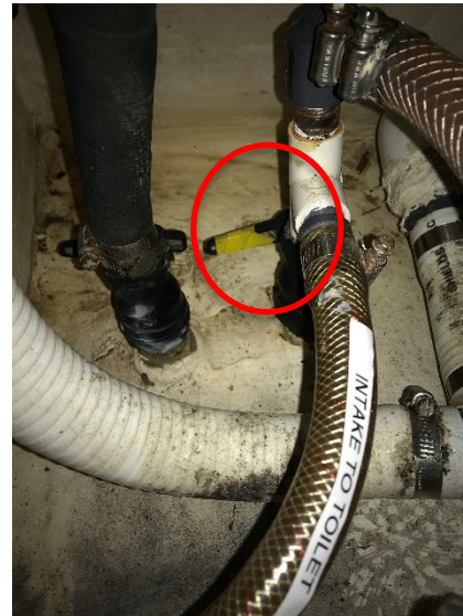
Thru Hull Handle for Toilet Intake
