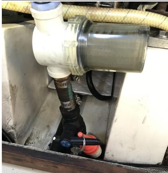
Sea Water Intake
